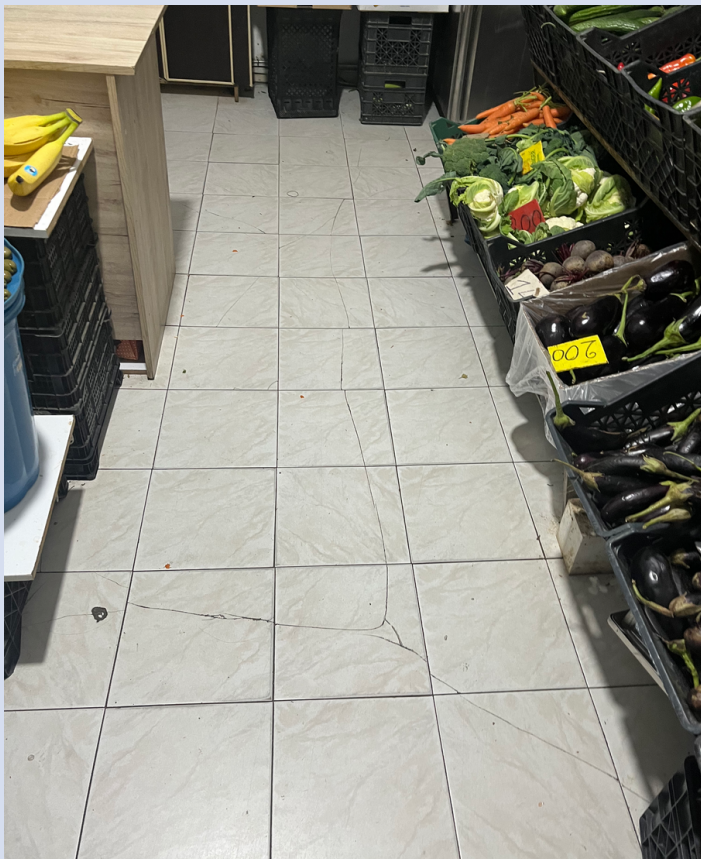
Figure 21: Minor tile cracks from the 2019 earthquake in a grocery store
