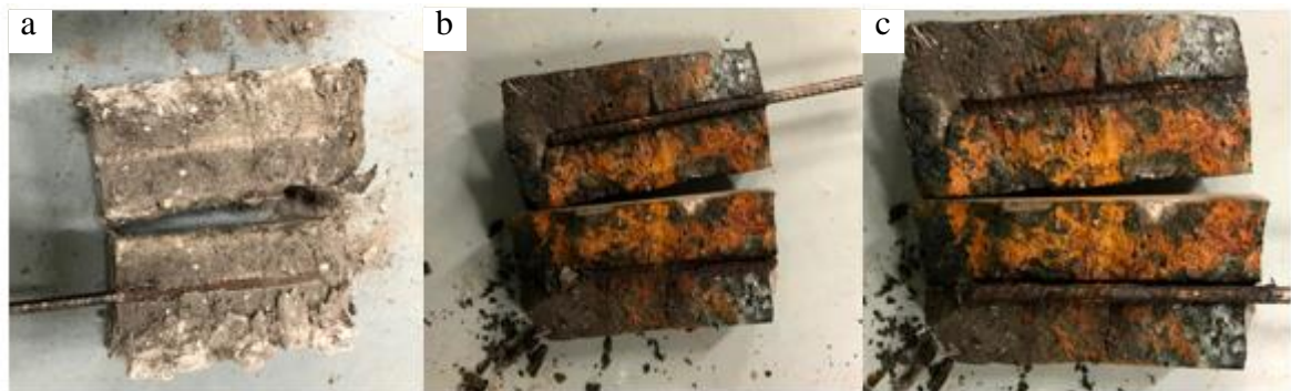
Figure 16: Cross section of samples after corrosion testing showing that the rebar reinforced concrete sample with plastic fibers (a) did not corrode unlike the glass (b) and steel (c) samples
