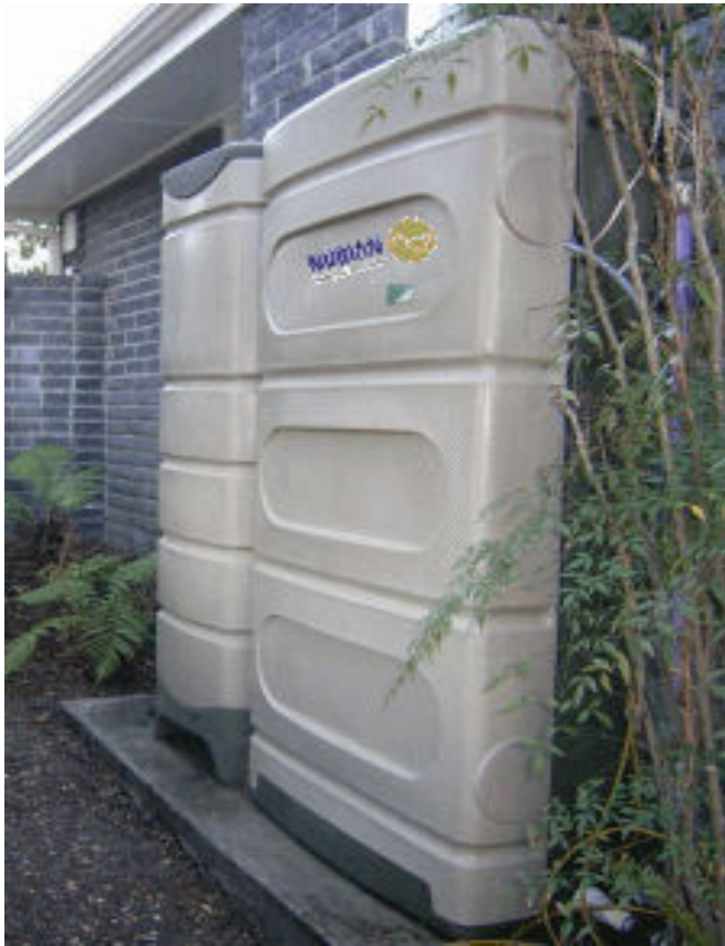
Figure 2-8: Nubian Greywater Storage Tank
