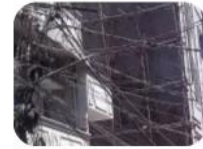
The Hans India (2020) Low cable wires [Photograph] https://www.thehansindia.com/news/cities/hyderabad/low-hanging-cables-put-people-in-a-state-of-tizzy-606288
