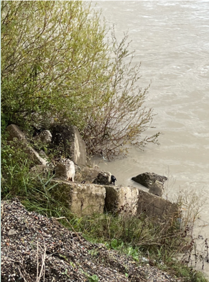
Figure 4.7: Degraded concrete structures placed by the municipality approximately 7 years ago.
