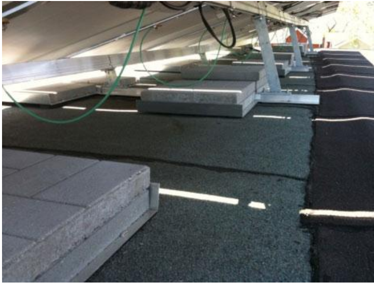
Figure 2: Photo of a ballasted array [8]
