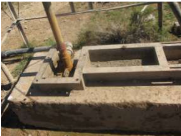
FIGURE 28: (LEFT) RUSTY PIPES
