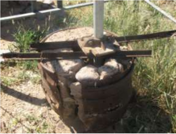
FIGURE 33: (LEFT) CRACKED BASE OF THE BOREHOLE
