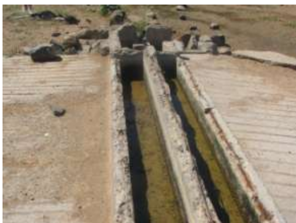
FIGURE 37: CONCRETE OF LIVESTOCK TROUGH IS IN POOR CONDITION
