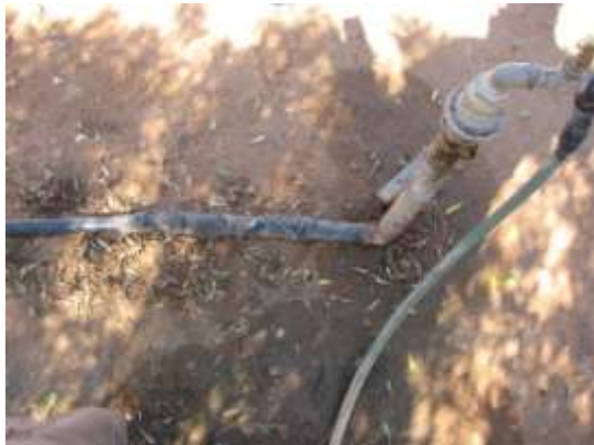
FIGURE 14: RUBBER PIPES THAT SUPPLY HOUSEHOLD TAPS ARE IN POOR CONDITION AND REQUIRE PATCHING
