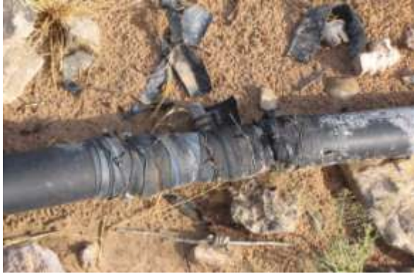
FIGURE 26: PIPING IS POORLY REPAIRED FROM THE SECOND RESERVOIR
