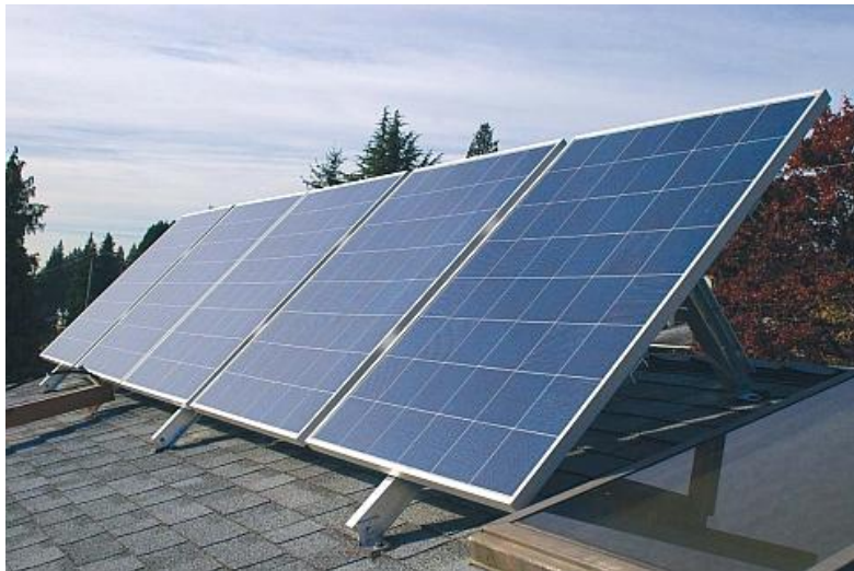
Sligo heating, roof-top solar panel
