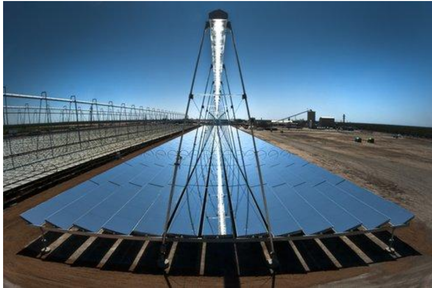
AREVA Solar's Compact Linear Fresnel Reflector technology at the company's Kimberlina Solar Thermal Power Plant in Bakersfield, California. (AREVA Solar) 33
