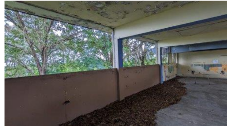
Figure 8: A building on the grounds of La Conde Community Center before being renovated into a usable space.
