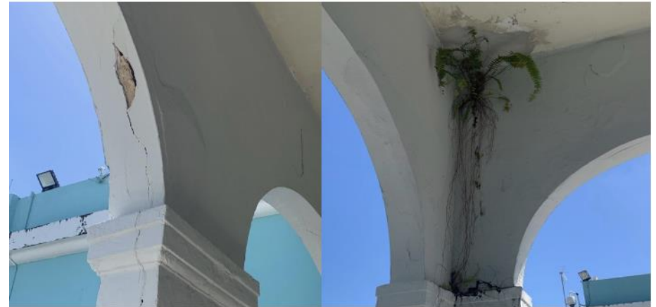
Figure 19 & 20: Cracked ceilings and plant overgrowth at La Goyco
