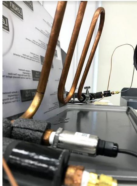
Figure 37: Evaporator with layer of condensed water
