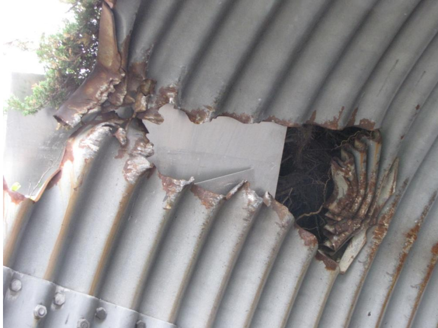
Figure 6 Structural Damage to the Tubes (Donovan, 2011)
