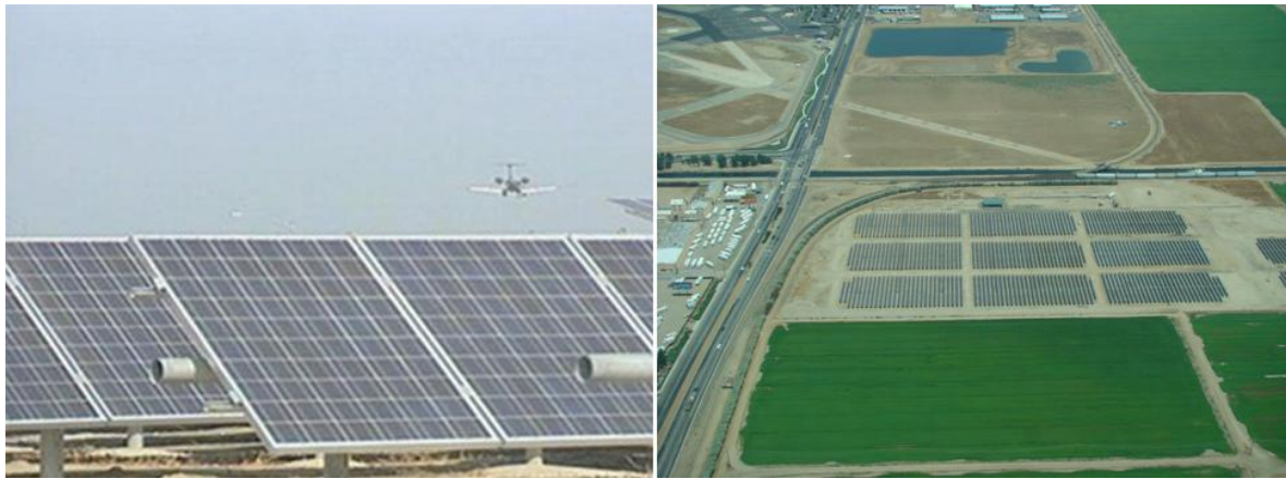
Fresno Yosemite Airport Solar Farm Information
