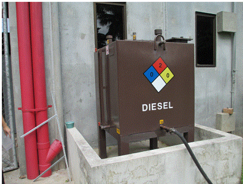
Figure 16: Diesel Storage Tank at Paquera Station
