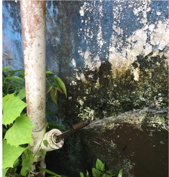
Figure 2.3.2: Leak at sand filter
