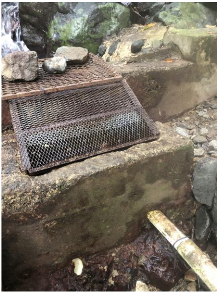
Figure 2.3.1: Grate Filter at beginning of water source
