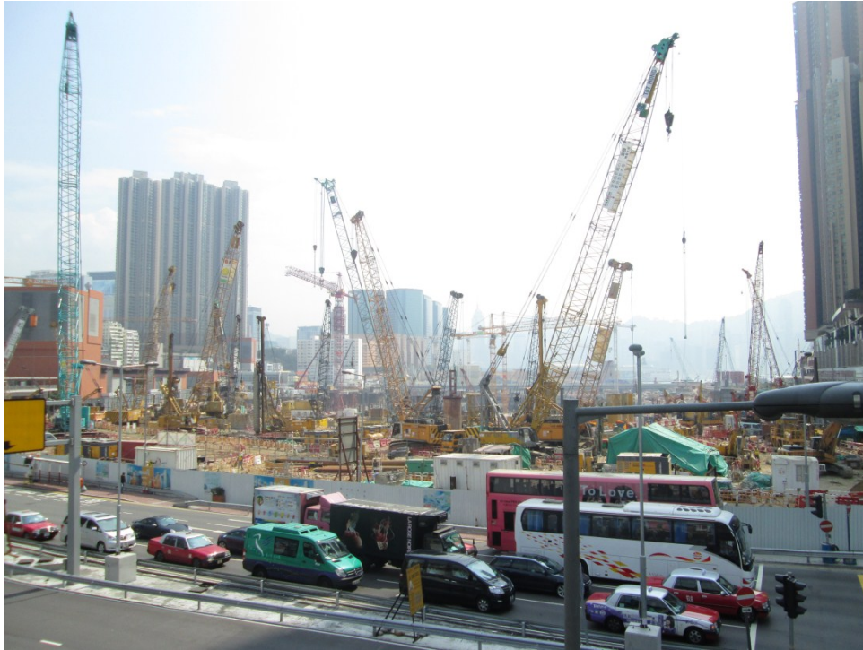
Figure 4: Construction along Austin Road, West Kowloon, site of one of Hong Kong's most recent land reclamation projects.
