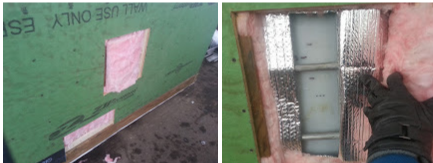
Figure 15: View of Access Panels
