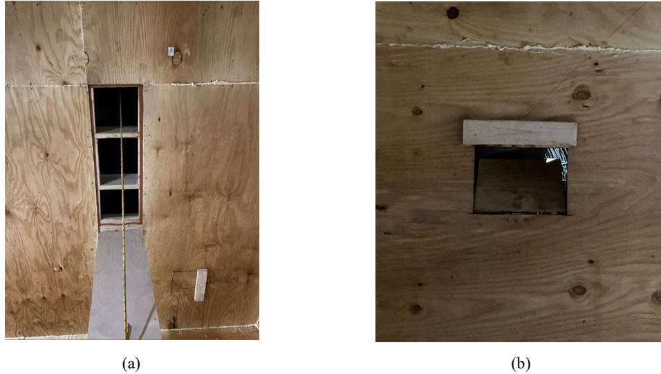
Figure 16: Picture of 36 x 111 cm buoyancy-driven flap (a) used to evacuate the combustion products pre-discharge on the full-scale enclosure ceiling. Picture of 9-by-12-inch forced convection vent (b) on the full-scale ceiling.
