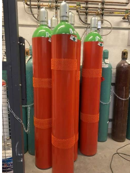
Figure 11: Picture of IG-100 tanks, red, next to type K tanks, green and brown, for scale.
