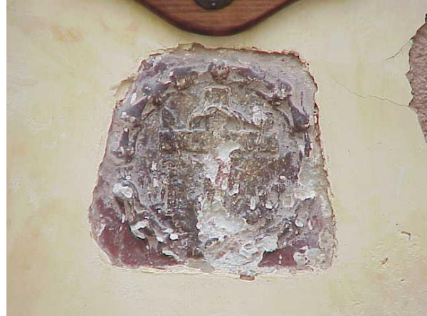
Figure 10: A deteriorated relief carving
