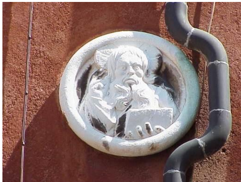
Figure 13: A pipe around a relief
