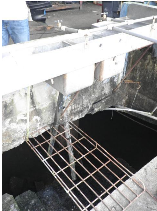
Figure 11: Sink drain at Puntarenas draining directly to ocean (Hayley Sandgren, 2011)
