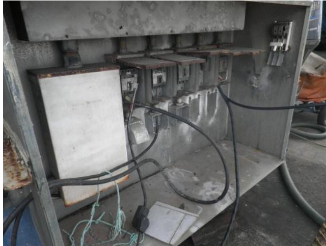
Figure 10: Exposed electrical junction box at Puntarenas (Hayley Sandgren, 2011)
