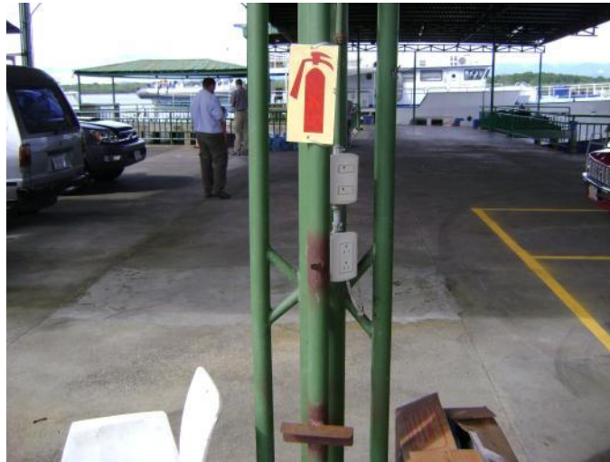
Figure 9: Fire extinguisher missing from its mount at port (Hayley Sandgren, 2011)
