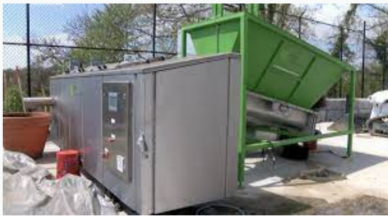
Figure 16: Cincinnati Zoo Aerobic Digester (Richard, 2021)
