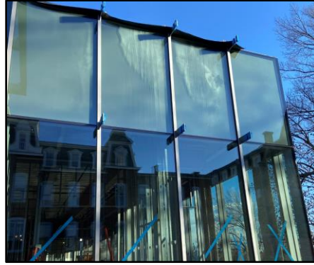
Figure 5.4: 01/07/21 Visible condensation in the shadowboxes (West elevation)
