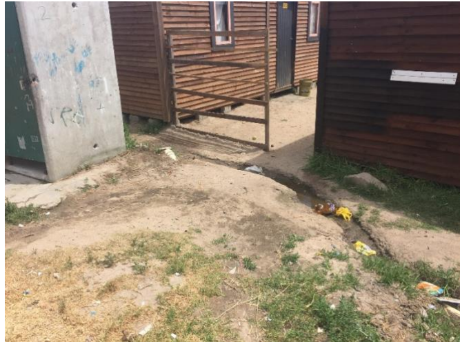
Figure 12: The sewage flowing from the broken ablution facilities next to Katriena's bungalow, on left, and Sabina's bungalow, on right.
