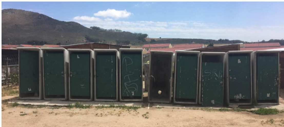
Figure 14: The vandalized ablution facilities that 10 families are expected to use in La Rochelle.
