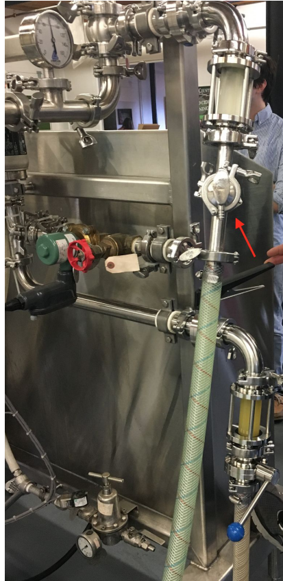
Figure 5: North Country Hard Cider's centrifuge control and tasting valves.
