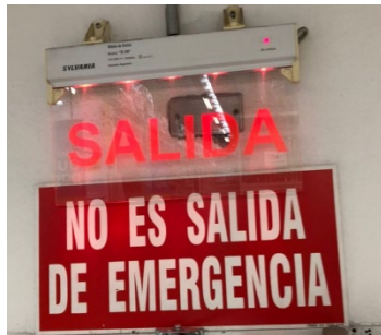
Figure 2. Contradictory exit signs, neither in accordance with NFPA 101 regulation.
