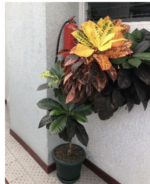
Figure 3. Fire extinguisher covered by plant, inhibiting accessibility
