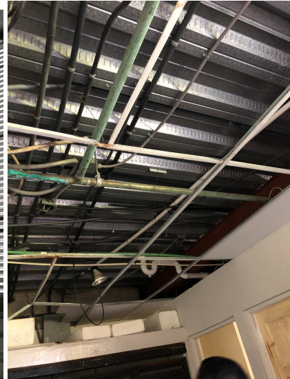
Wall does not go from floor to ceiling slab, enables fire to travel between even fire-rated rooms
