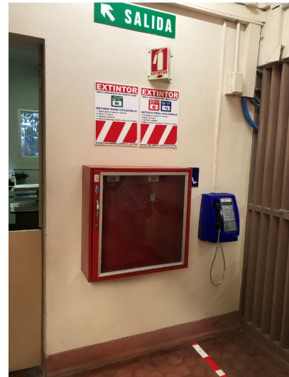
Figure 12. Missing Fire Extinguisher (By Authors)
