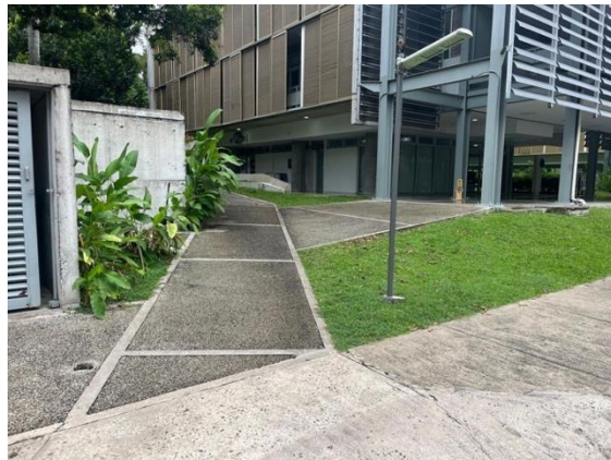
Non-ADA Compliant Ramps at CdS Dormitories
