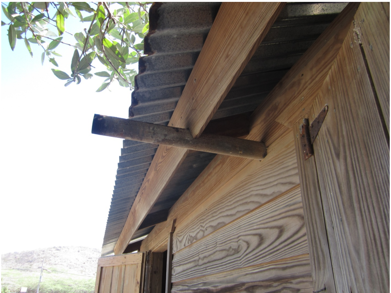
Figure 29: Exposed Exhaust Pipe of Current Motor System
