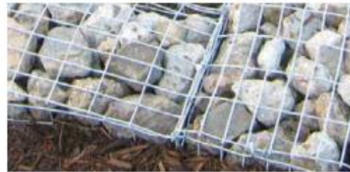
Figure 25: Overfill rock into gabion and seal tight to prevent sagging. Rock will settle over time.
