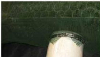
Figure 18: Cut "X" in Biaxial Mesh and Geotextile to accommodate outlet pipes and seal with stainless steel band clamps
