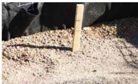
Figure 22: Place biofiltration soils, being careful not to mix with any other site soils, to specified depth
