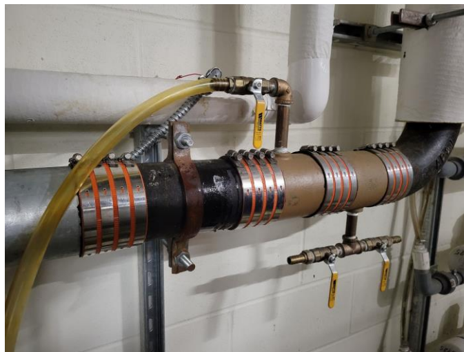
Figure 8: East Hall Gray Roof Stormwater Collector
