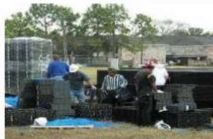
Figure 3: Assembling on site during excavation will increase speed once the excavation is completed
