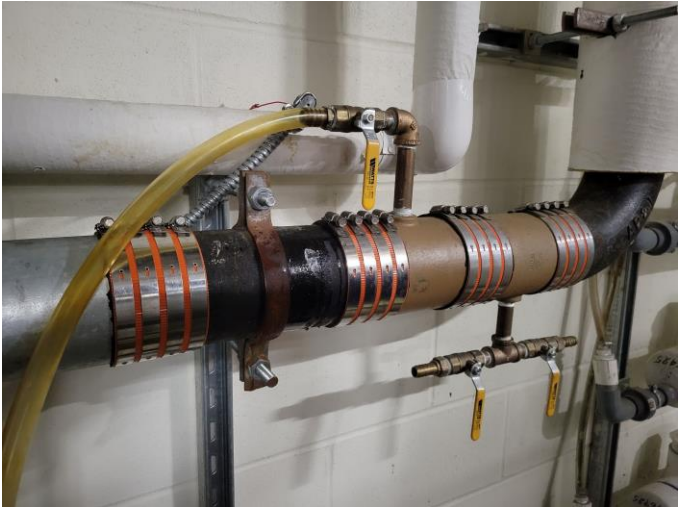
Figure 8: East Hall Gray Roof Stormwater Collector
