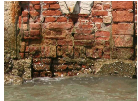
Figure 12: Damage to Building Foundation Resulting from Moto Ondoso (see footnote 15 for source)
