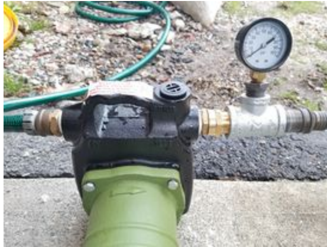
Figure 21: Pressure gauge attached to threaded tee on pump outlet;
