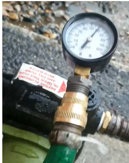
Figure 22: Pressure gauge attached directly to hose outlet
