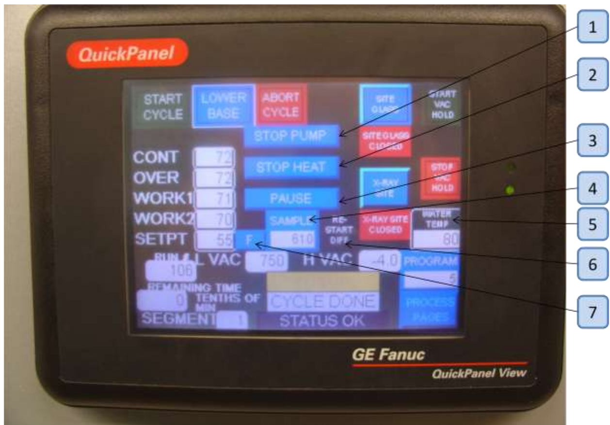
Figure 6: Upgraded PLC for IA Unit
