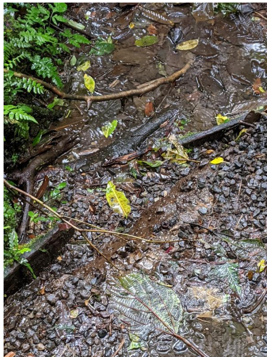
Figure A21. Trail Border, Encantado: Trail border is damaged, causing erosion and loss of structure and gravel on trail.
