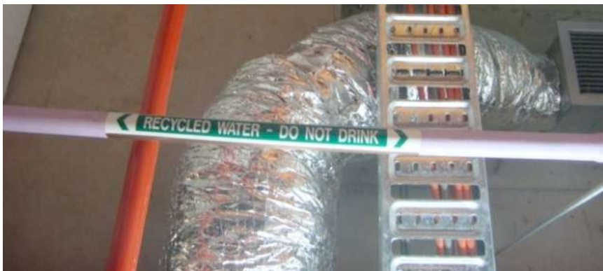
Figure 30: Pipe circulating recycled water in the shower rooms
