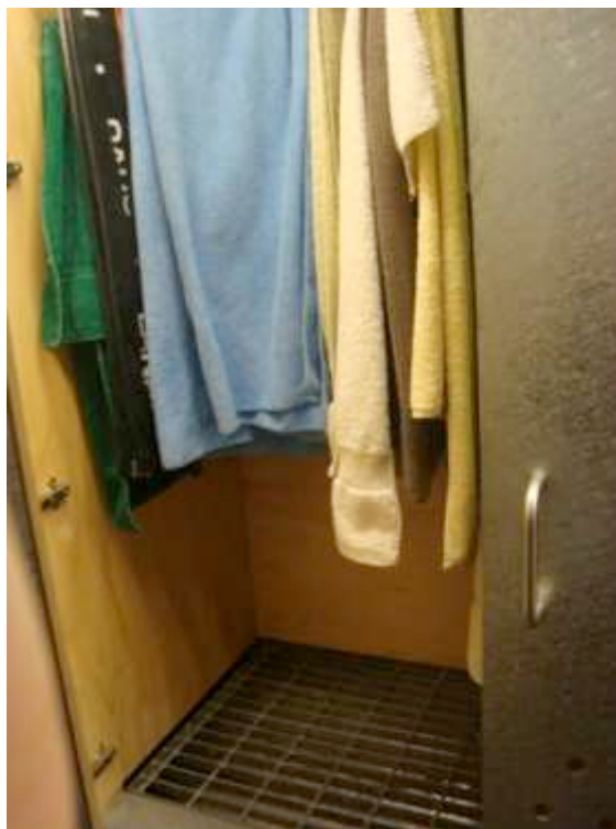
Figure 28: Towel closet for employees that blow air through the vents to dry them
