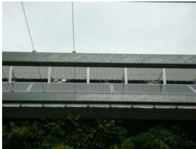
Figure 36: Solar panels on roof
