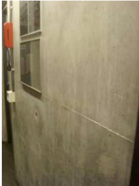
Figure 31: Unpainted walls that do not release harmful pollutants and needs very little maintenance
