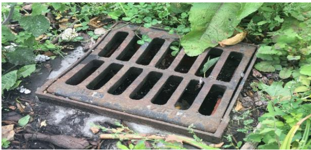
Figure 24: Gully in rain garden.
