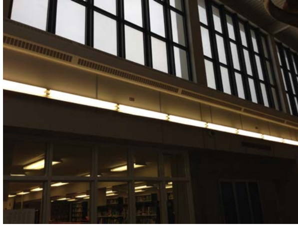
Figure 27: Main Corridor Lights
