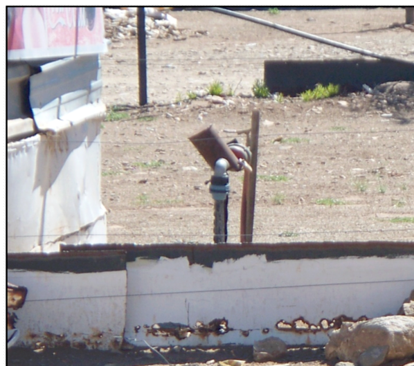
Private Standpipe at a Residence in the Informal Settlement
