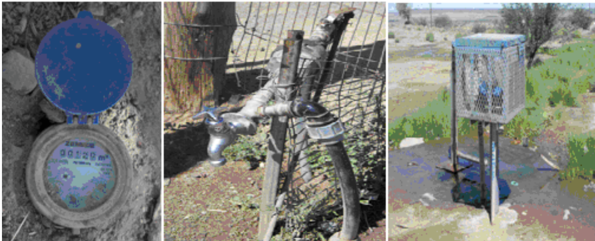
FIGURE 13: DELIVERY METHODS TO USERS (FROM LEFT TO RIGHT) CONVENTIONAL METER, YARD TAP, STANDPIPE
