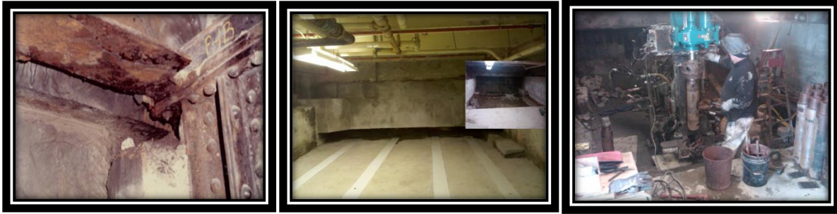
Figure 14: Pictures of structural damage from inside the Coast Guard Building (left: corroded header beam, middle: spandrel beam retrofit, right: drilling activity for beam support)
