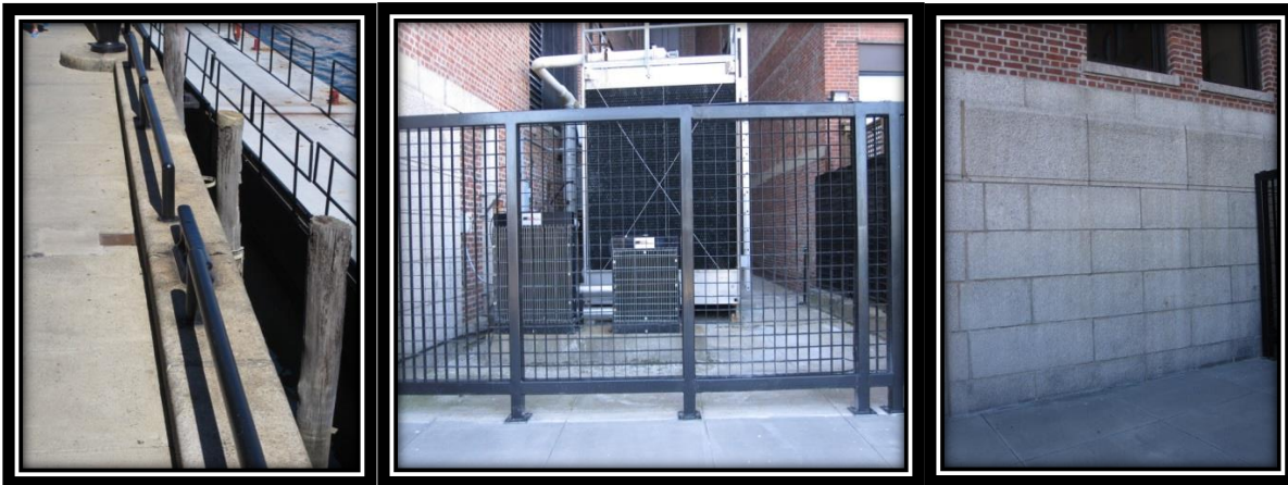
Figure 15: Pictures taken of the vulnerable features of the Coast Guard Building (left: seawall outside of building, middle: outdoor HVAC and electrical equipment, right: height of first floor)
