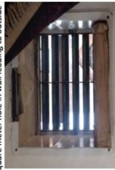
4 Really Bad Square meter hole in wall leading to outside
