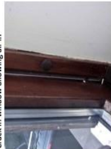
3 Bad Crack in window allowing air in
