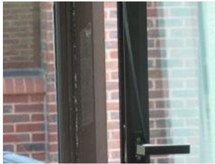
Figure 3: A window that had a seal falling off it. This is possibly an area for improvement.
