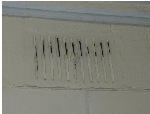
Figure 1: Ventilation duct needing to be insulated
