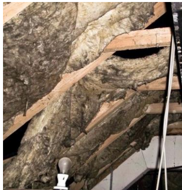
Figure 4: Insulation falling off the roof
