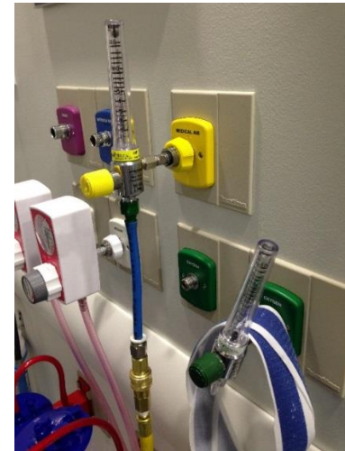
Figure 0.6 Medical air connection
