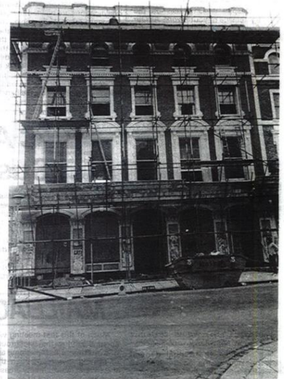
Above: Restoration on The Winch in progress. (Photo Roger Perry) Below left: Supporters of the project on holiday in Mull, Scotland. (Photo Graham Good)
