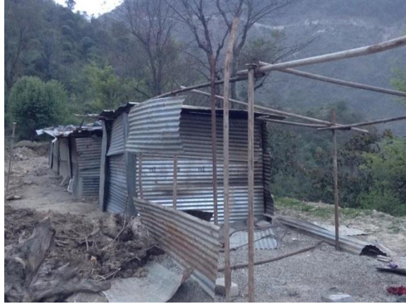
Figure 2. Tin structure destroyed by wind.
