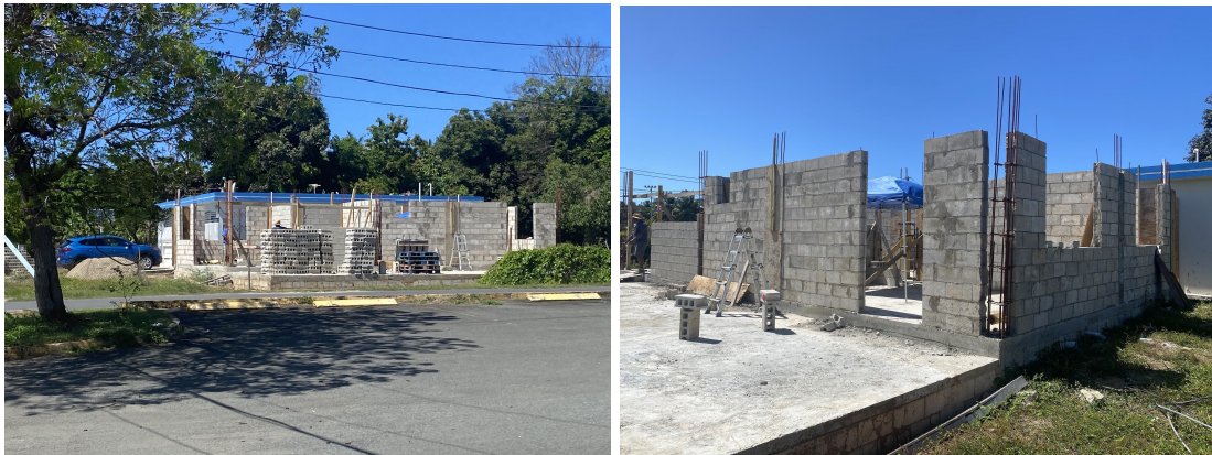
Figure G: Photo taken by team members of the construction progress from across the street (Left). Photo taken by team members of the construction progress up close (Right).
