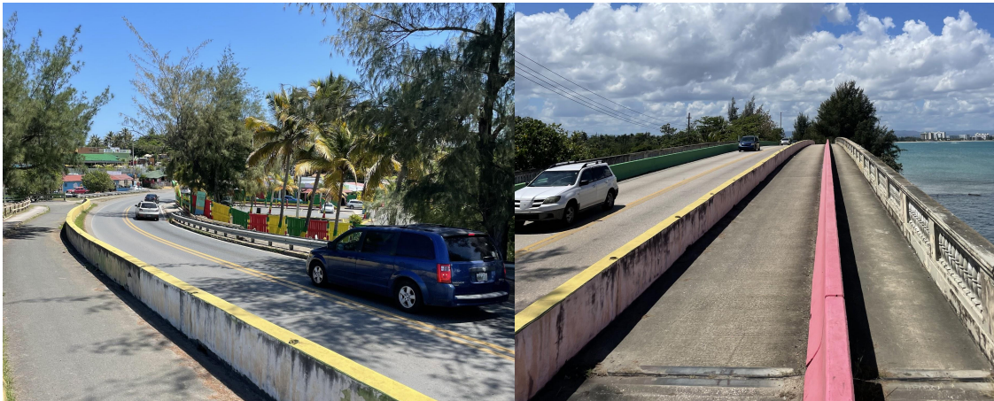
Figure D: The only road that leads to Loíza from San Juan. (April 2022)
