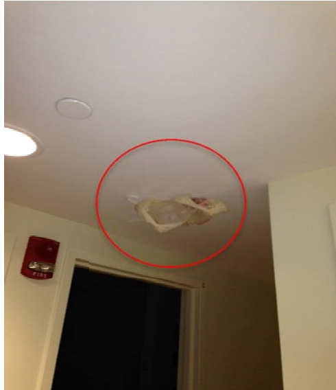
Figure 45-Smoke detector workaround devised by students due to poor ventilation and localized smog (Residence Hall-EH)
