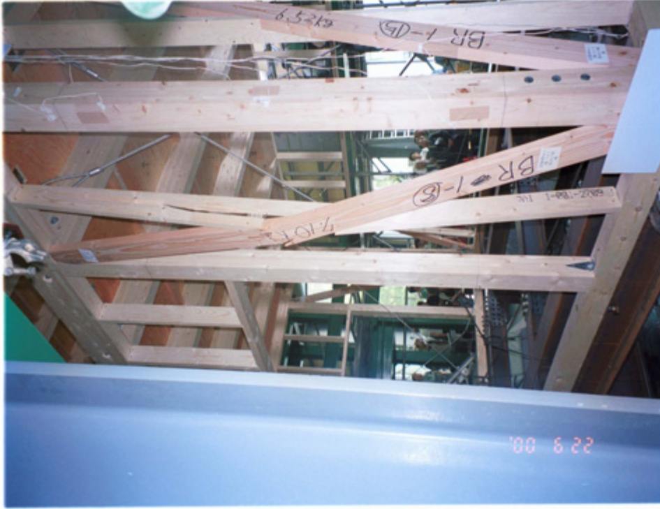
Figure 8.3.2. A damaged wooden brace occurred during the test run at the load level 3.50m/s 2 . A secondary damage occurred in the stud connected to the damaged brace. (from Shimizu et al; 2000).
