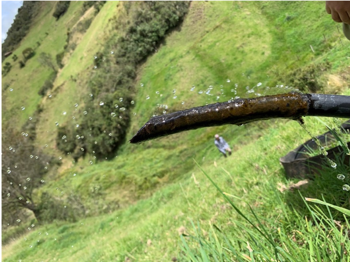
Figure 4.4: A Leaking Capitation Point
