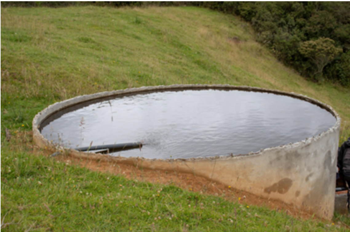
Figure 2.11: The Tank ETAPA Implemented
