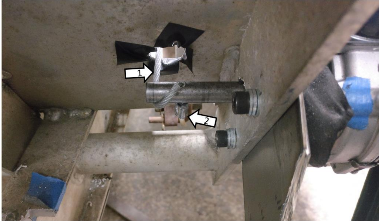
Figure 54: Shows the brake cable (Item 1) wrapping around the shaft of the brake motor. Item 2 is the crimp on the end of the cable keeping it secure.
