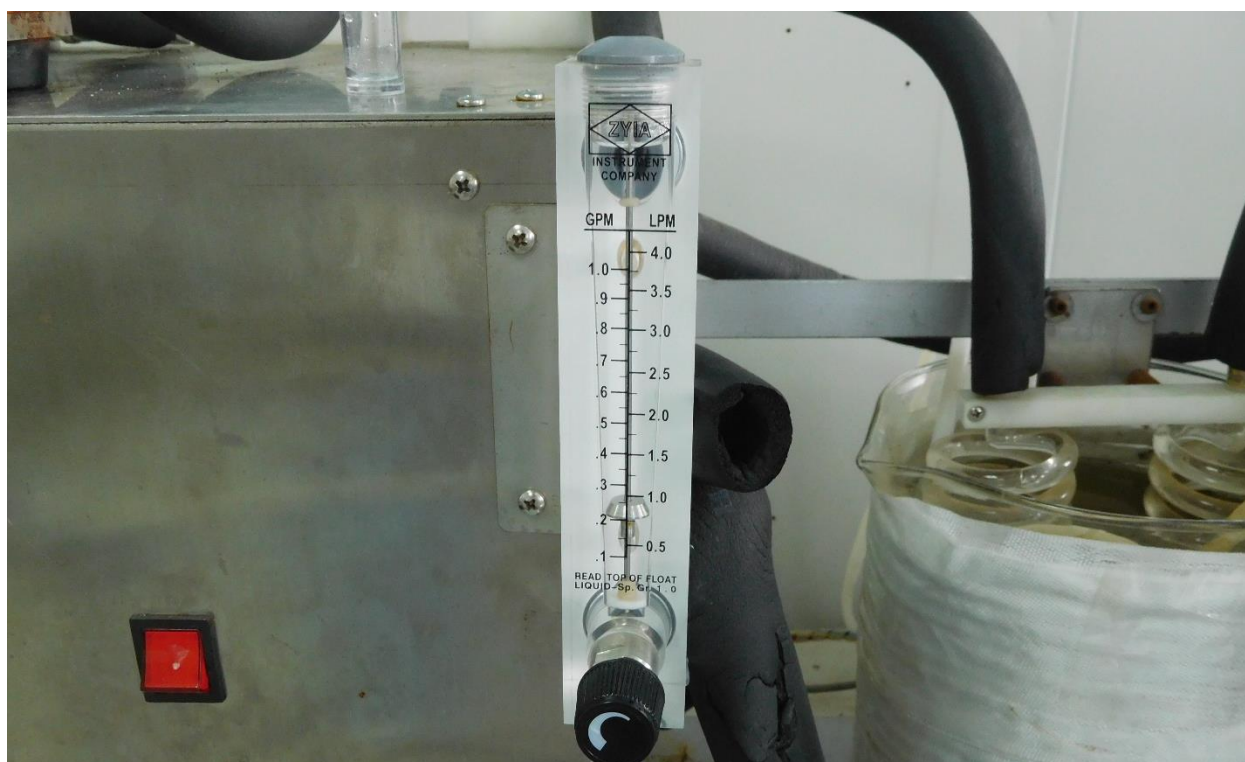
Figure A8: Right flow meter which controls flow of permeate stream.
