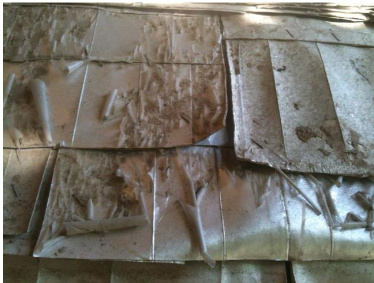
FIGURE 11: PEELING POLYETHYLENE ON ORIGINAL TETRA PAK ROOF
