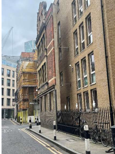
Figure 3: Example of a facade in which the historic outer wall was preserved with new construction occurring behind it. Located on the corner of Gun St. and Artillery Lane in London, England, UK.
