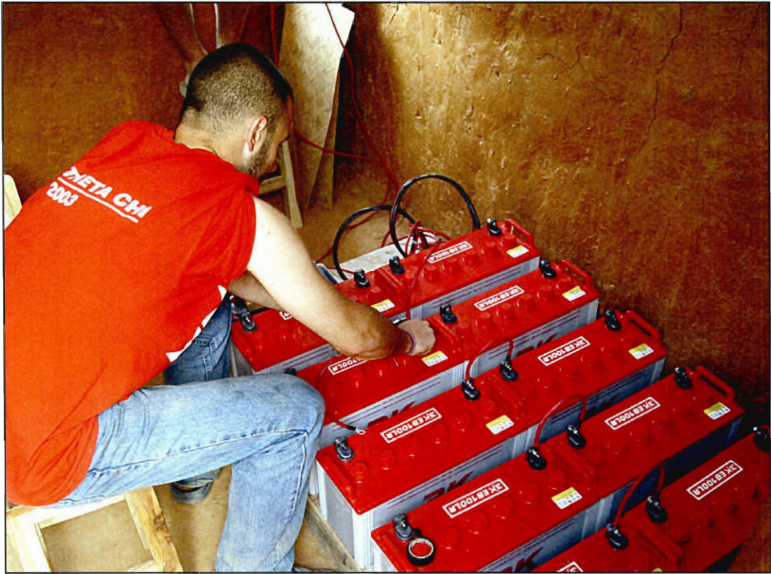
Figure 12: Wiring of the battery array
