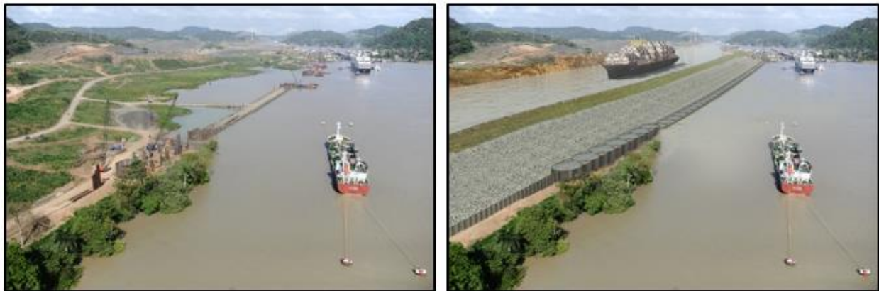
Figure 9: Cofferdam and earth dam during construction and rendering of after construction (Autoridad del Canal de Panamá, 2015)
