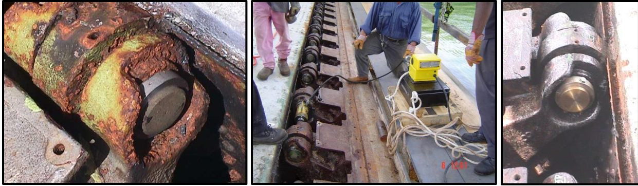
Figure 47: Corrosion on the hinges and the pin replacements (Chen & Cano, 2003; Autoridad del Canal Panamá, 2004)
